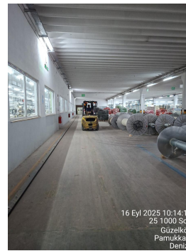
NC-Fuel Combusting Forklift in Closed Area.jpg
