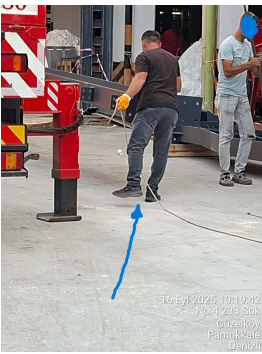
NC-Contractor Employee without Protective Shoe.jpg
