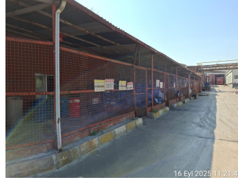
Waste Storing Area.jpg
