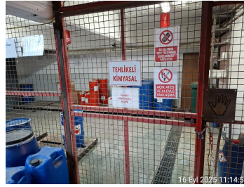
Hazardous Chemical Storinng Room.jpg
