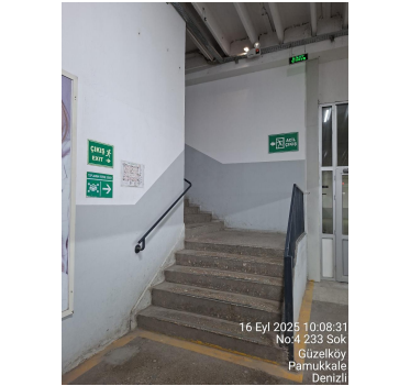
Emergency Escape Direction Signpost.jpg
