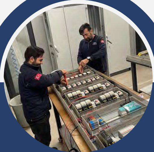
Automate programmable (PLC)
